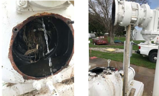
Images of sludge pump at sewer plant.
