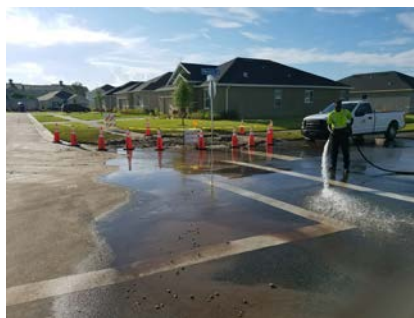
Image of road clean up after water main break.
