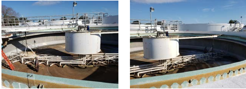
Images of clarifier at sewer plant.
