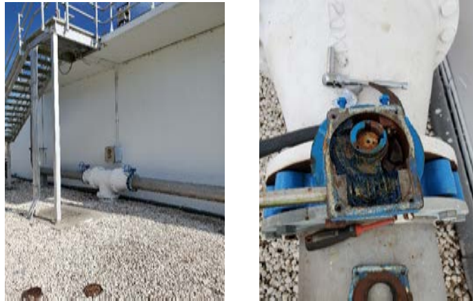
Images of digester and airline valve.
