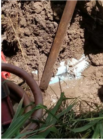
Image of water main break.
