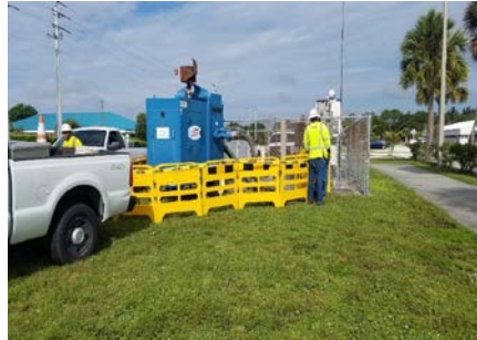
Image of Meadowlane lift station.
