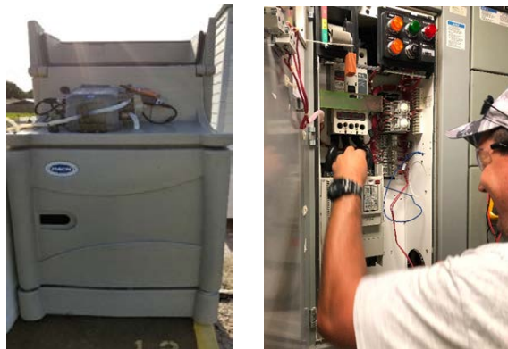
Images of controller and installation at sewer plant.
