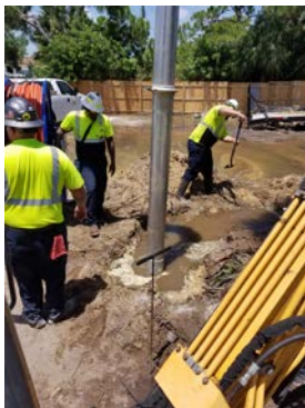
Image of City employees repairing a water service break on Ellis Road.
