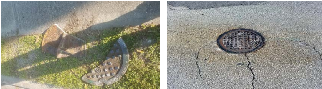
Images of broken and replaced manhole cover on U.S. 192.
