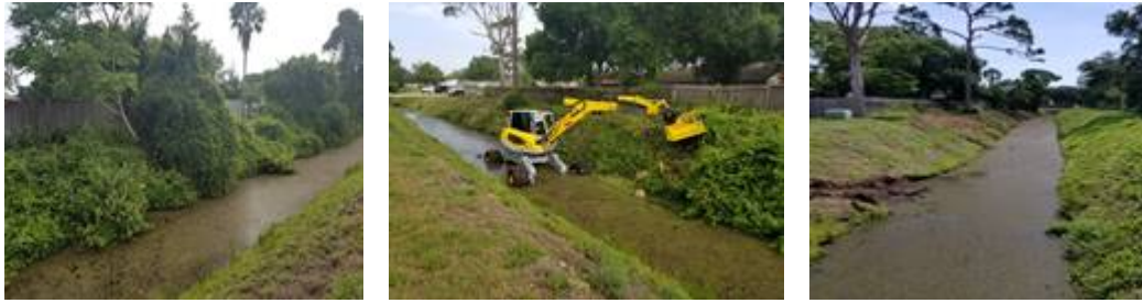
Images of before, during and after the Menzi Muck cleaned and de-mucked the C-5 canal in Clements Woods.
