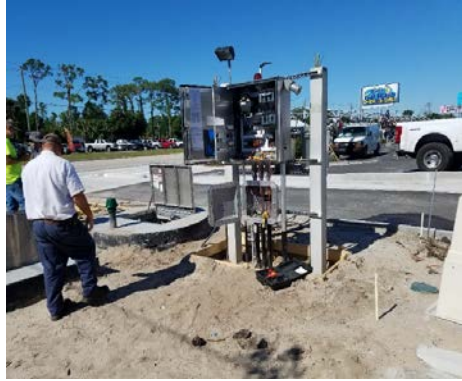
Image of lift station at Bill's Car Wash on U.S. 192.
