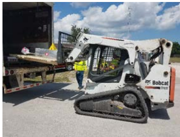
Image of control panel being delivered to plant.
