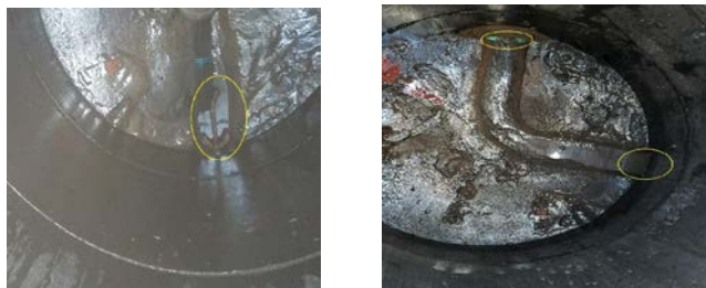
Images of plug in manhole at Cypress Landing.
